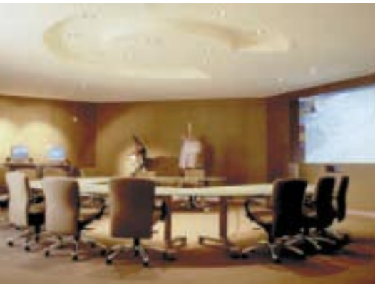
Lighting is activated via a combination of manual switching and automatic control by Photoelectric and Movement Sensors.
