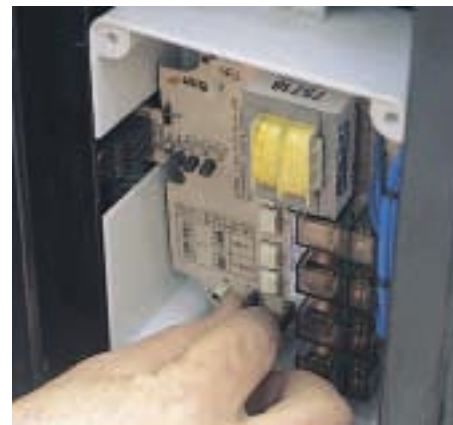
Due to size restraints inside each tower, four channel relay units were customised.
